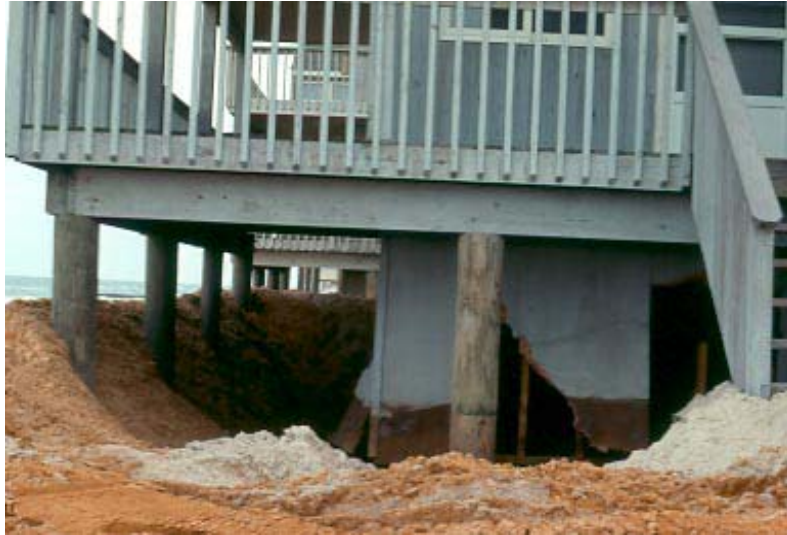
Figure 1. Damage to breakaway walls under an oceanfront house in Brant Beach, Long Beach Island, as a result of a storm in December 1992. Note hole in wall facing the viewer and buckle in wall out to the ocean side due to hydrostatic load (Photo courtesy of Dr. Susan D. Halsey).
