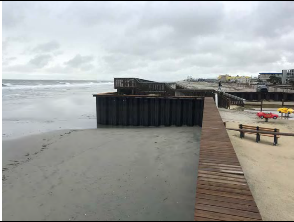
Photo #9 – View of timber cap and steel bulkhead looking southwest toward 7 th Avenue.
