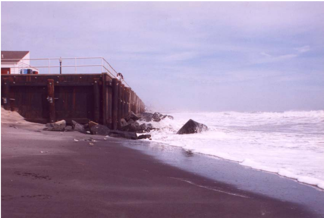
Figure 57. Timber bulkhead at Bradley Beach, New Jersey under direct wave attack. Note rock placed at the base of the structure to prevent scour (Photograph by Dr. Thomas O. Herrington).
