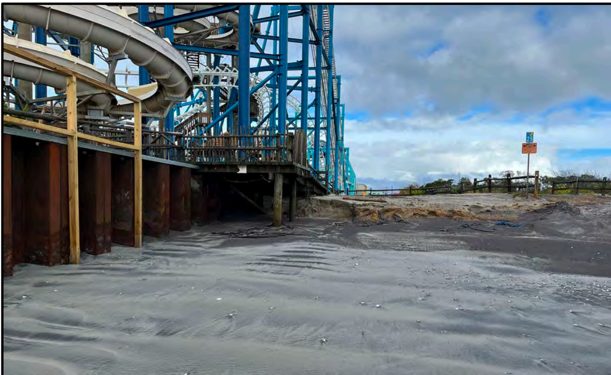
PHOTOGRAPH 2. View west of the eroded and scoured public accessway at the 25 th Avenue beach access terminus.
