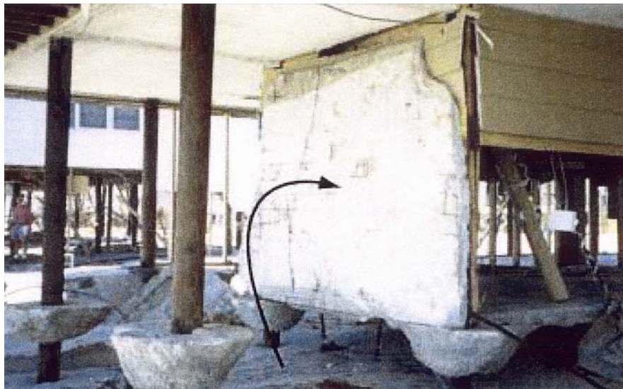
Figure 26. Scour around pilings and under on-grade slab. Notice that the slab broke free of the pilings and flipped up vertically. Poured concrete under a pile supported structure can generate unexpected loads on the structure, if undermined like above. Reprinted with permission from the FEMA Coastal Construction Manual (FEMA, 2000).
