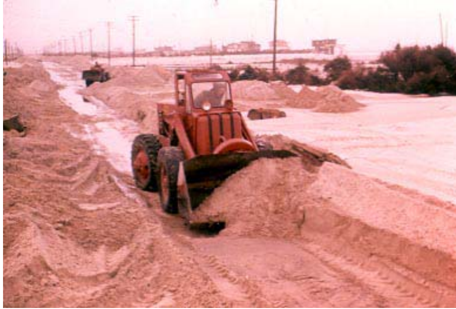
Figure 20. Front end loaders removing extensive storm washover from Long Beach Boulevard, New Jersey, in the Loveladies section of Long Beach Island. At some locations, washover was over four feet deep (Photo courtesy of Lawrence Wagner).
