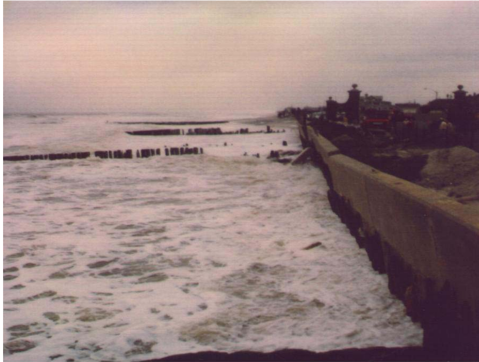
Figure 32. Concrete retaining wall, originally constructed to prevent wind blown sand from depositing on Ocean Avenue, in Belmar, New Jersey, under direct wave attack during the October 31, 1999 northeaster (Photograph by Dr. Michael S. Bruno).
