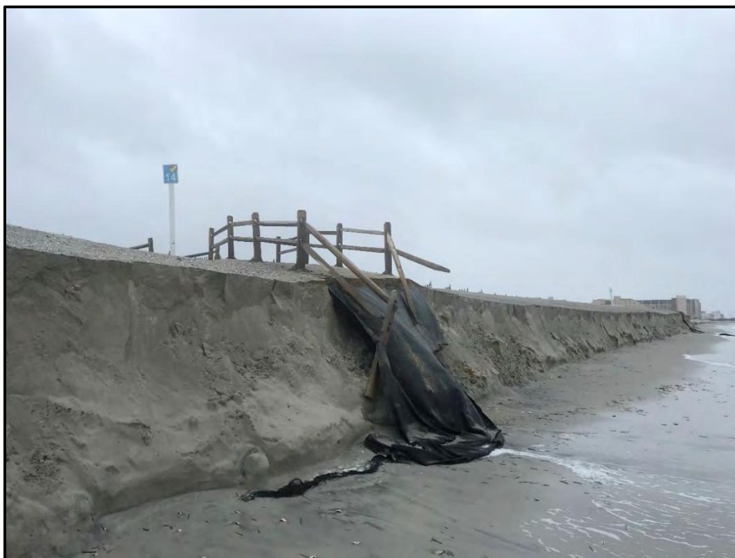
PHOTOGRAPH 2. View north of the dune scarp at the 14 th Avenue beach access path. Note that the beach berm has been eroded which has caused normal high tides to impede on the toe of dune.
