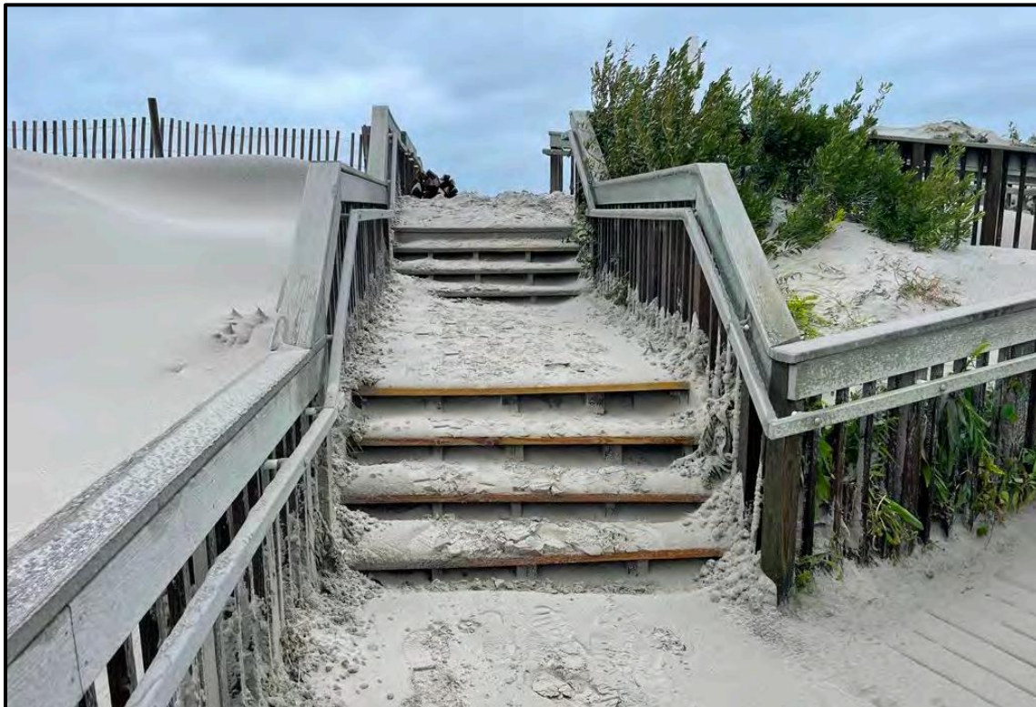
PHOTOGRAPH 6. View of the dune walkover and ADA access ramp in front of the City of North Wildwood Beach Patrol headquarters. This access path has sustained significant damage since the passage of hurricane Ian in early October 2022. It is anticipated that the remnants of this structure will need to be removed, particularly as the risk of failure increases.
