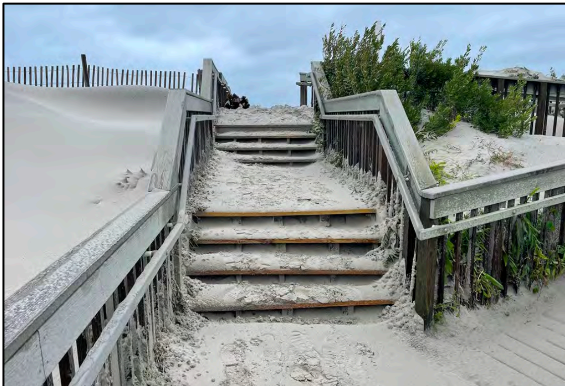
PHOTOGRAPH 6. View of the dune walkover and ADA access ramp in front of the City of North Wildwood Beach Patrol headquarters. This access path has sustained significant damage since the passage of hurricane Ian in early October 2022. It is anticipated that the remnants of this structure will need to be removed, particularly as the risk of failure increases.
