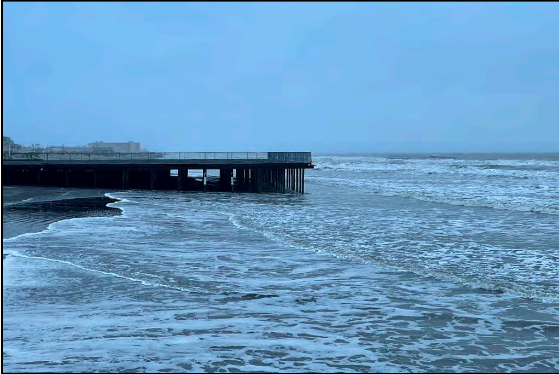
PHOTOGRAPH 7. View north of the 24 th Avenue pier terminus and absence of beach berm waterward of the pier end, which precludes the sand backpassing truck route.
