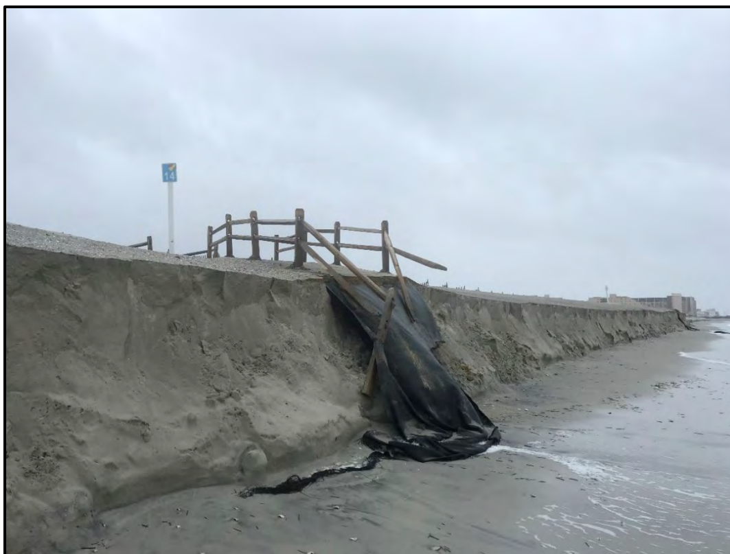
PHOTOGRAPH 2. View north of the dune scarp at the 14 th Avenue beach access path. Note that the beach berm has been eroded which has caused normal high tides to impede on the toe of dune.
