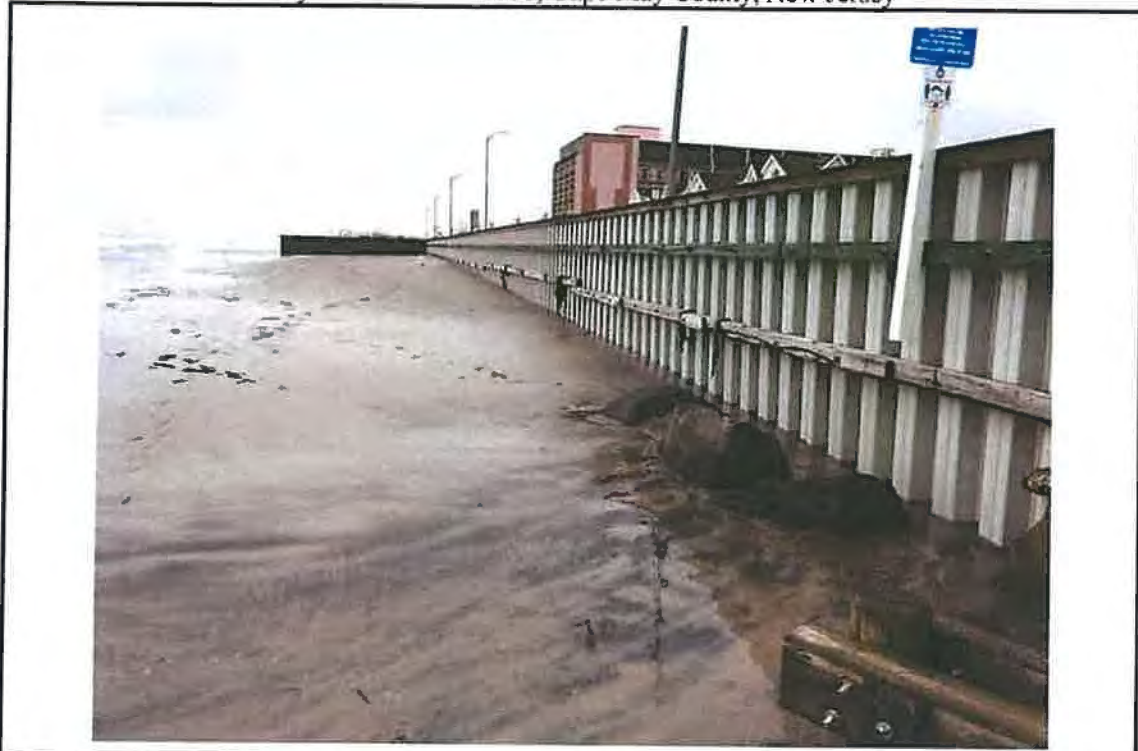
Photo #3 – View of waterward side of vinyl bulkhead at 3 rd Avenue looking southwest.
