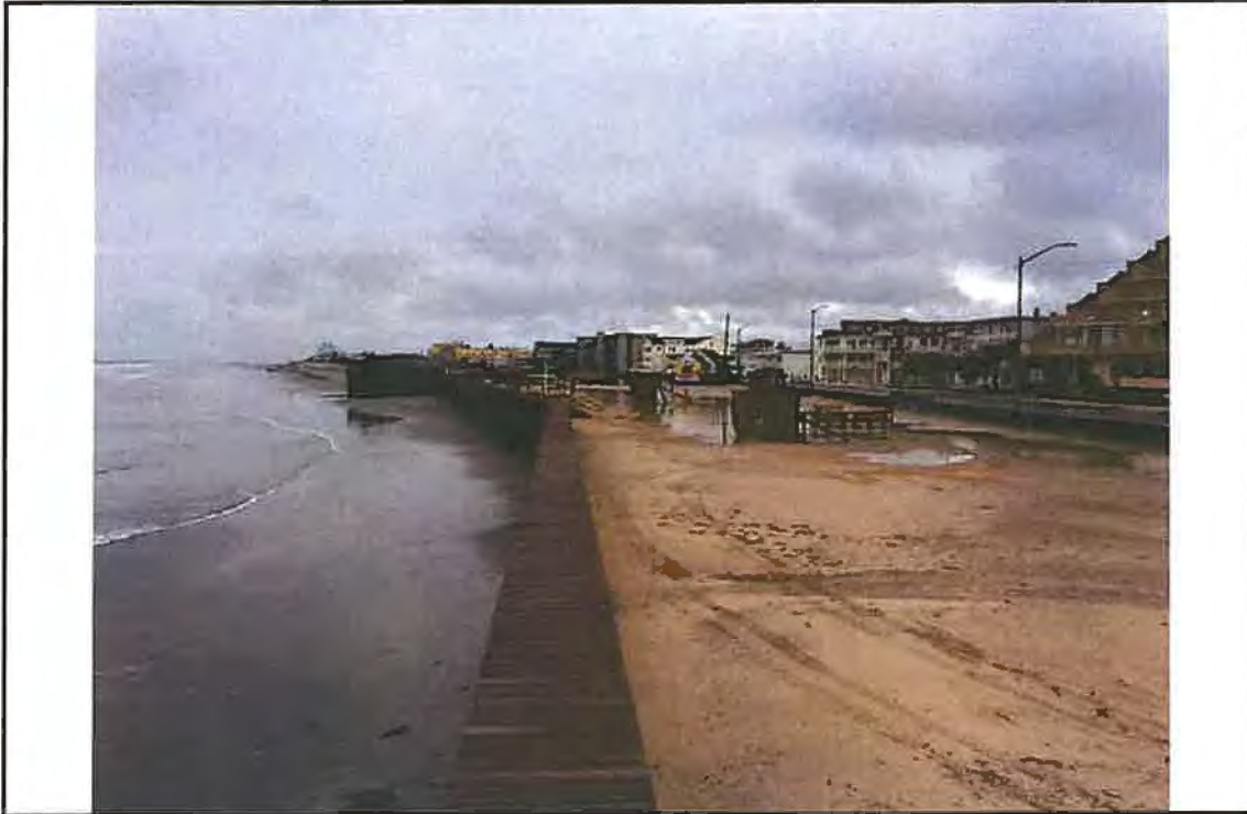
Photo # 7 – View of timber cap and steel bulkhead at 6 th Avenue looking southwest.
