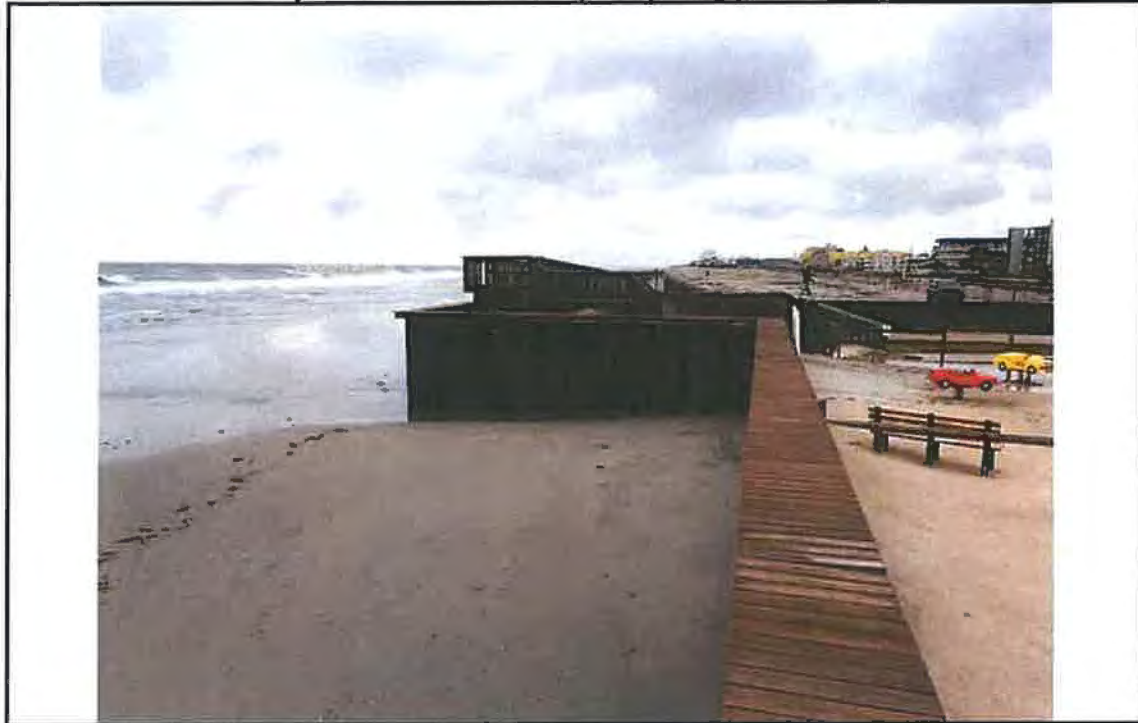
Photo #9 – View of timber cap and steel bulkhead looking southwest toward 7 th Avenue.
