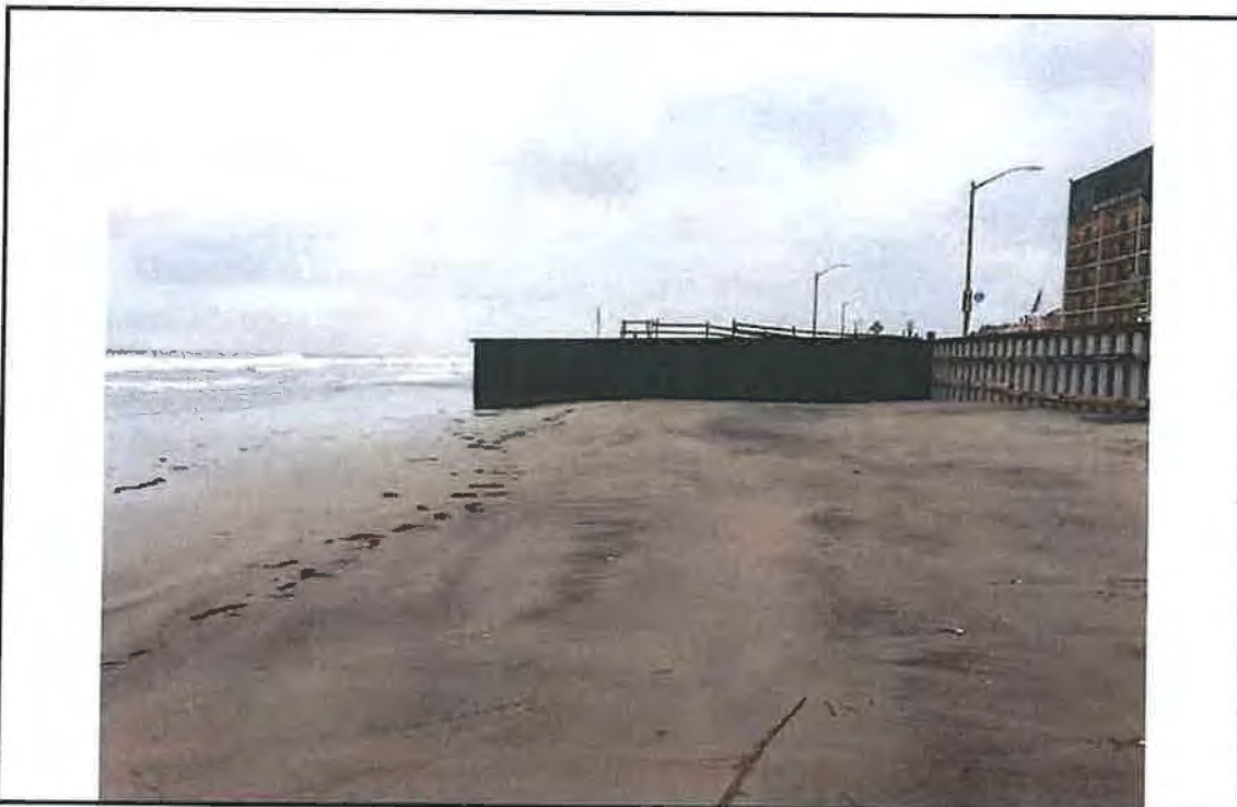
Photo #4 – View of waterward side of vinyl bulkhead and steel bulkhead, and former dune area at 4 th Avenue looking southwest.
