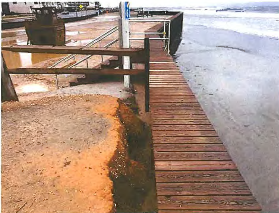
Photo #8 - View of steel bulkhead at 7th Avenue looking northeast showing erosion and flooding on landward side of the bulkhead.
