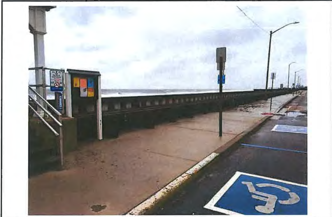
Photo #1 – View of landward side of vinyl bulkhead at 3 rd Avenue looking southwest.
