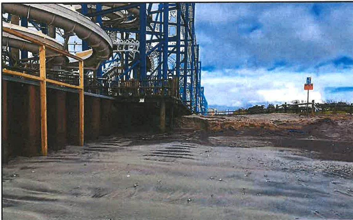
PHOTOGRAPH 2. View west of the eroded and scoured public accessway at the 25 th Avenue beach access terminus.
