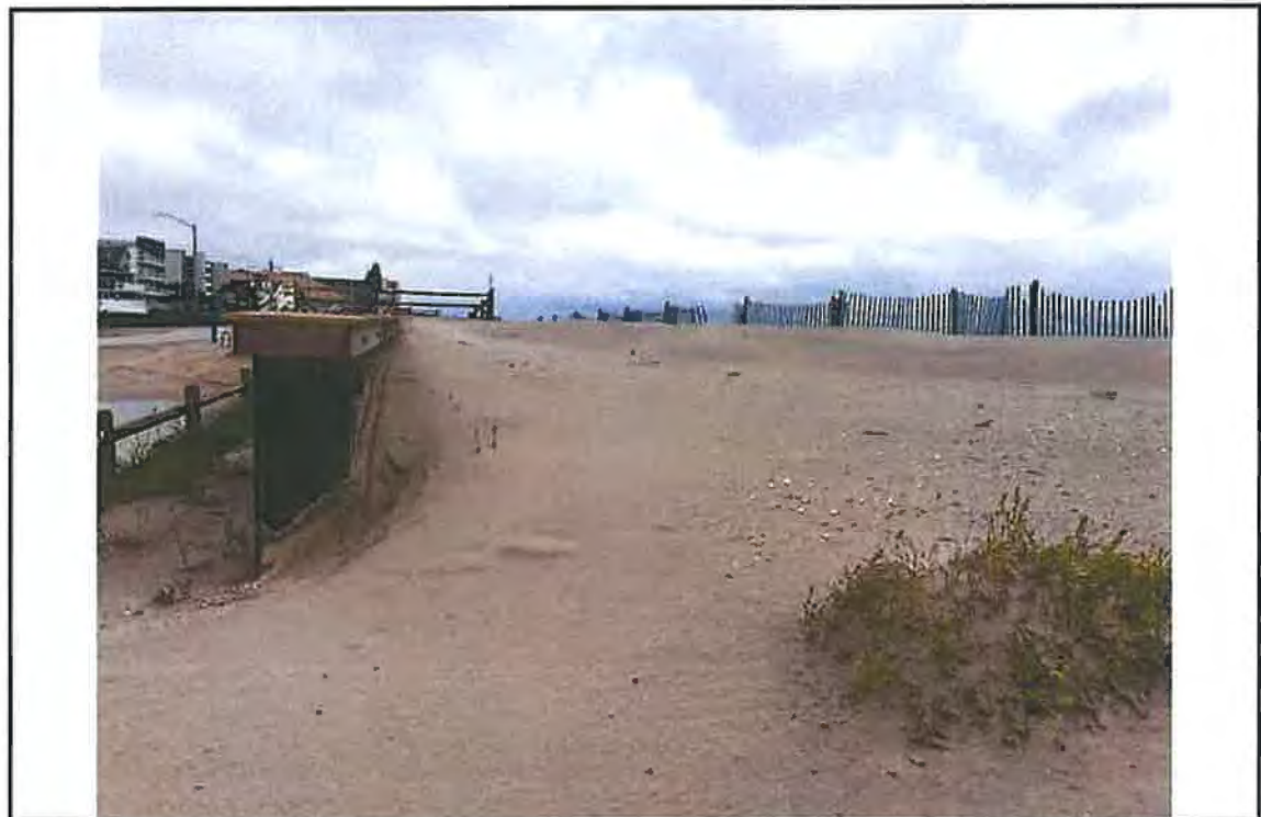
Photo #16 – View of steel bulkhead and location of former wetland at 13 th Avenue looking northeast.
