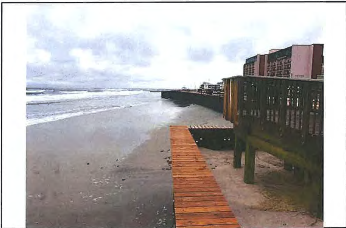
Photo #10 – View of timber cap and steel bulkhead at 7 th Avenue looking southwest.
