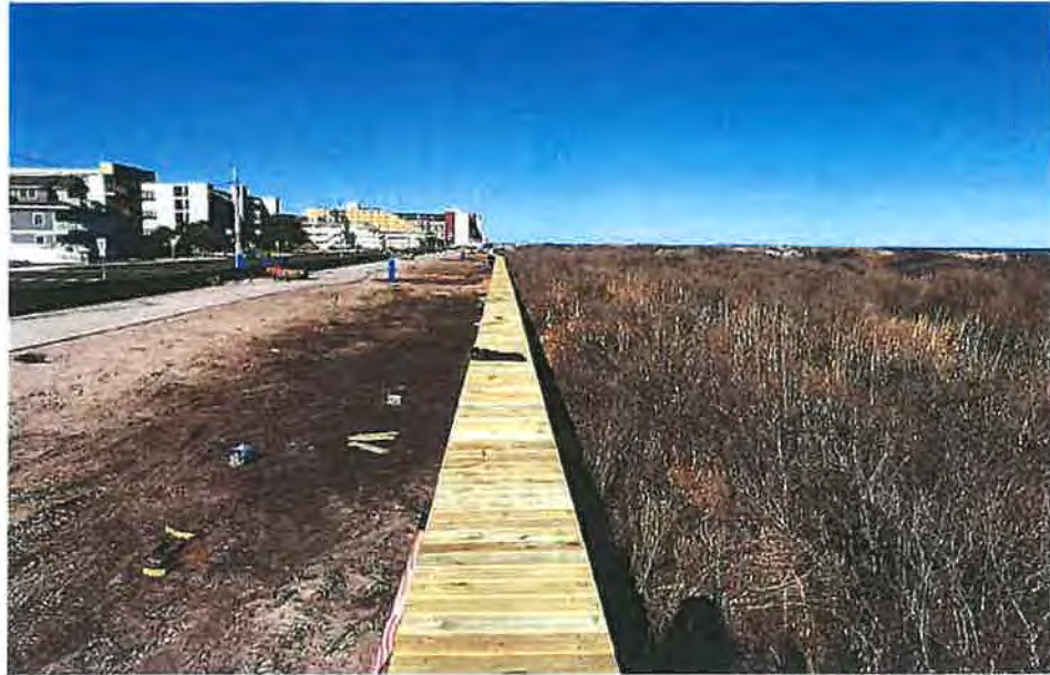
(Exhibit E, 2020 Photograph showing installation of a bulkhead.) The bulkhead (center) does not disturb the dune located on the righthand side.
