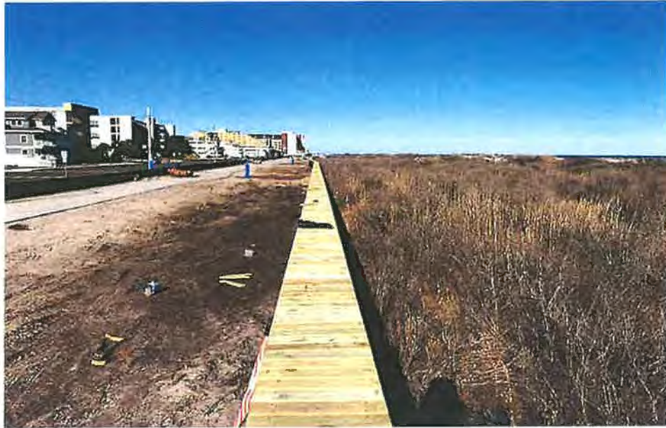
(Exhibit E, 2020 Photograph showing installation of a bulkhead.) The bulkhead (center) does not disturb the dune located on the righthand side.
