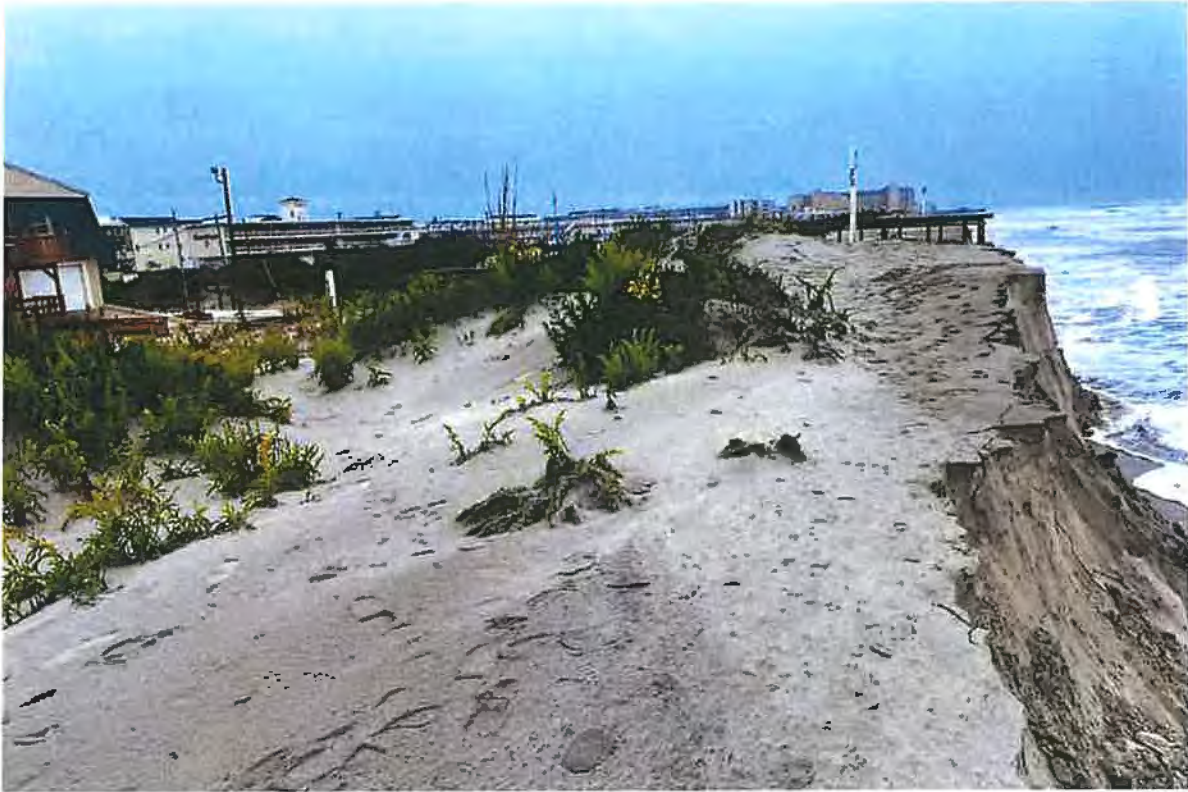
(Exhibit A. View of severe dune scarping located directly in front of the City of North Wildwood Beach Patrol Building between 15 th and 16 th Avenues.)
