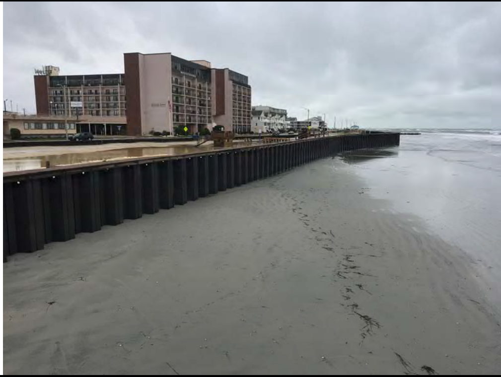
Photo #11 – View of waterward side of steel bulkhead at 7 th Avenue looking northeast.
