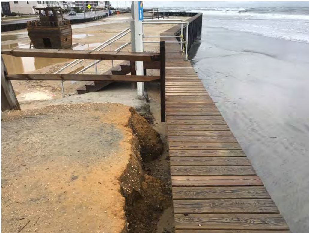
Photo #8 - View of steel bulkhead at 7th Avenue looking northeast showing erosion and flooding on landward side of the bulkhead.
