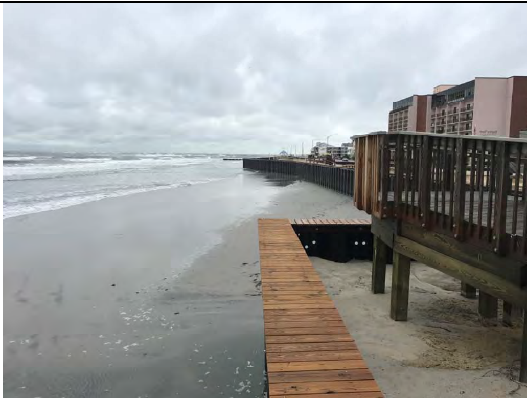
Photo #10 – View of timber cap and steel bulkhead at 7 th Avenue looking southwest.
